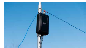
Wire antenna installation example
